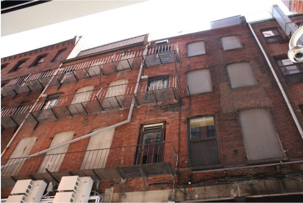
Figure 20. Gridley Street elevations of 123-127 and 129-131 Pearl St. Photograph by Wendy Frontiero, June 2023.
