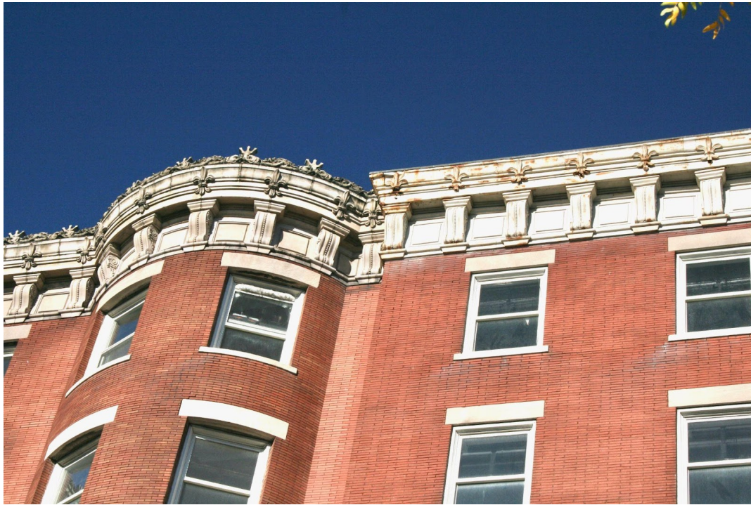
Figure 8. Entablature detail, Brookline Avenue elevation: 1897 (left) and 1902 (right). October 2022.
