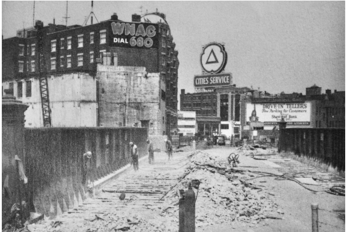
Figure 20. View northeast on Brookline Avenue toward Kenmore Square during demolition of the old Brookline Avenue bridge over the New York Central (Boston & Albany) Railroad (summer 1963). Hotel Buckminster is on the left, bearing a wall sign for radio station WNAC. Construction of a new bridge to span the Massachusetts Turnpike Extension raised the street grade on Brookline Avenue.
