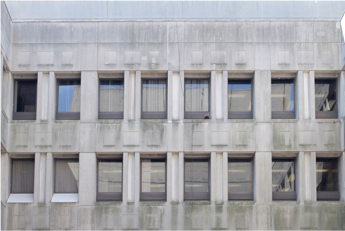
Courtyard at sixth and seventh floors, north-facing facade—representative soiling conditions on precast concrete sections (May 23, 2018).
