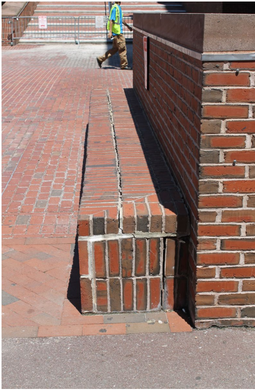
Top: General masonry failure adjacent to accessible ramp to the west entry (May 23, 2018).
