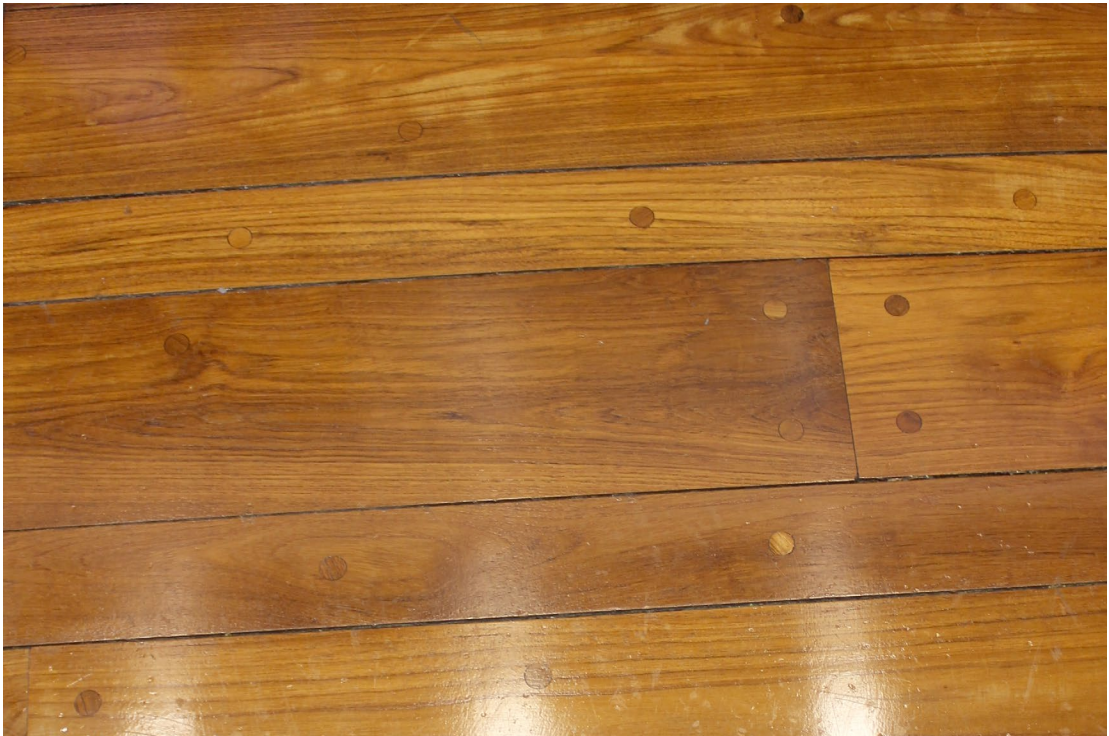
Wood floor, mayor's office showing plugged fastening holes (June 21, 2018).
