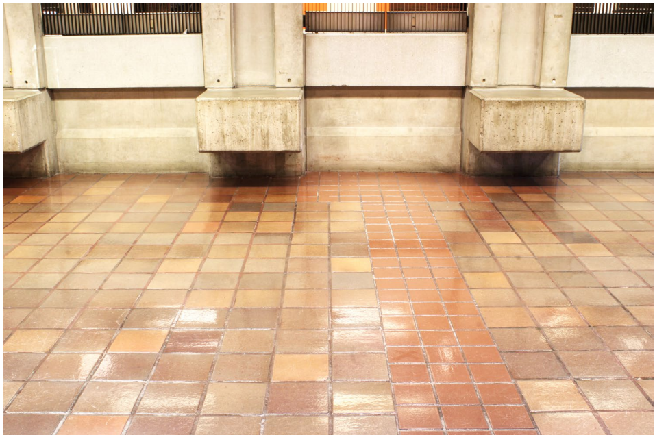
Clay tile showing a section replaced with an off-the-shelf material (January 11, 2021).
