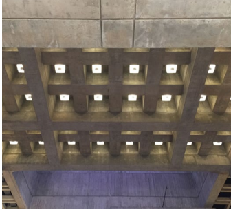
New LED fixtures in the plaza lobby.
