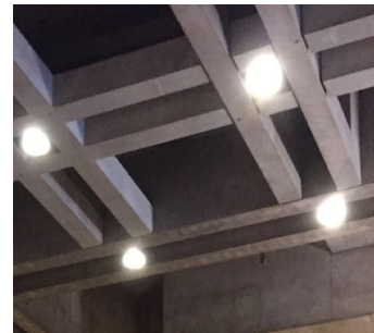
Incandescent can downlights in the transaction area.
