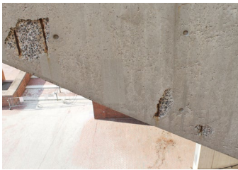
Top: Crazing located outside of council chamber at fire stair balcony (March 29, 2018).
