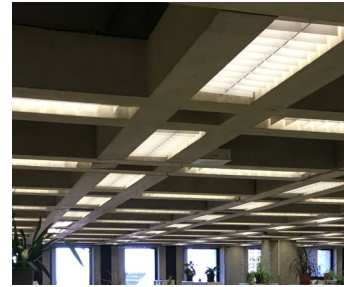
Fluorescent fixtures in an administrative office space.
