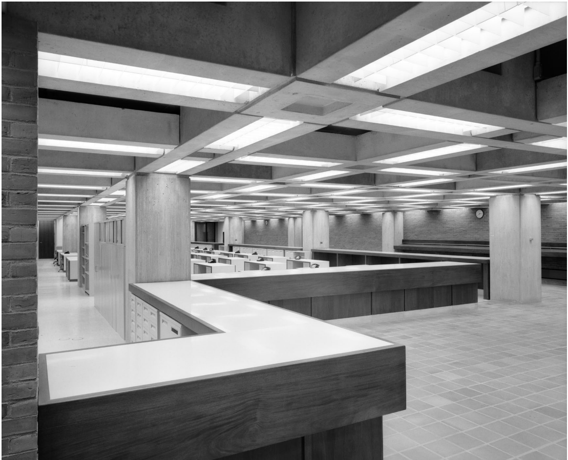
Linear fluorescent fixtures in a second-floor office space.
