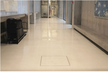
Polyester terrazzo floor on the fifth floor’s known delamination area (June 21, 2018).
