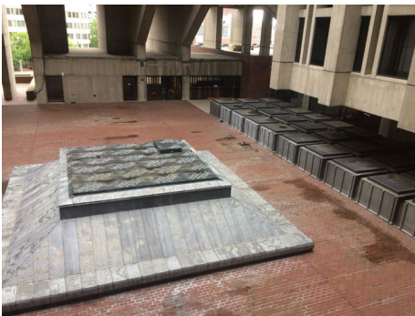
View of central skylight showing metal cladding and Grace I&W covering the top opening.
