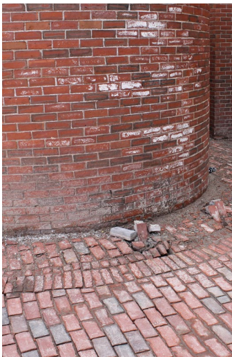
Top: Displacement cracking (May 23, 2018).
