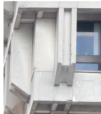
East elevation at south corner (nominally above mayor's office suite); note multiple instances of spalled concrete on fins and window sills (June 21, 2018).
