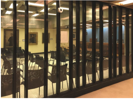
Meeting room 801, showing the storefront system that does not match the original.
