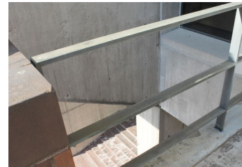
Original exterior railing detail; fire escape area adjacent to city council chamber (June 21, 2018).
