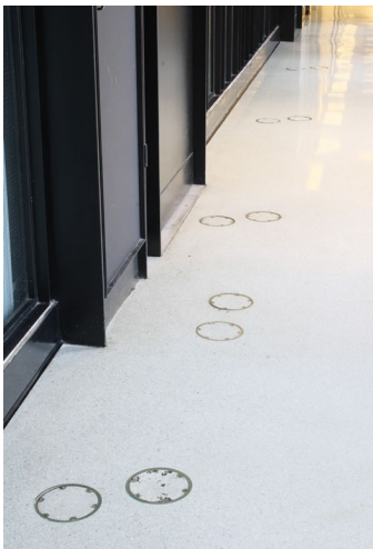
Walker duct covers in floor.
