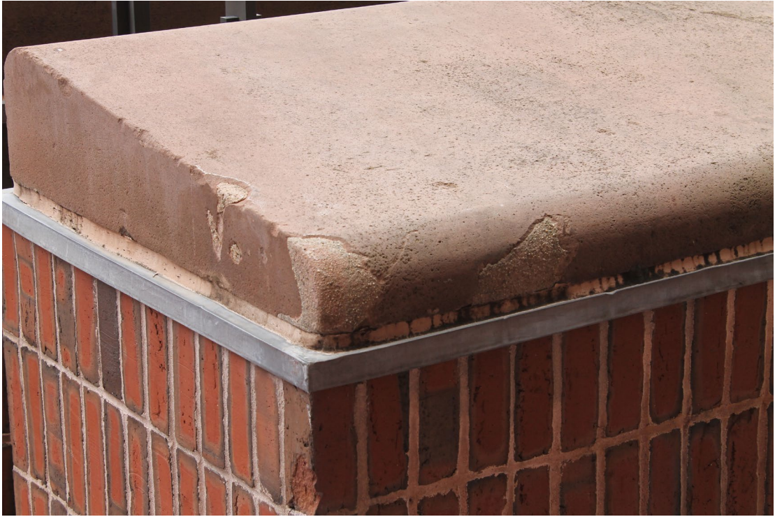
Poorly matched brownstone repairs and through-wall flashing detail (May 23, 2018).
