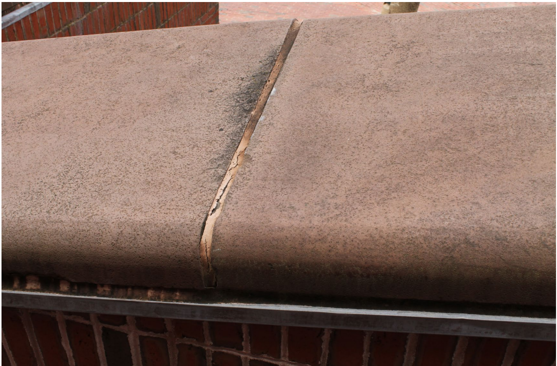
Brownstone with sealant mortar joint (May 23, 2018).
