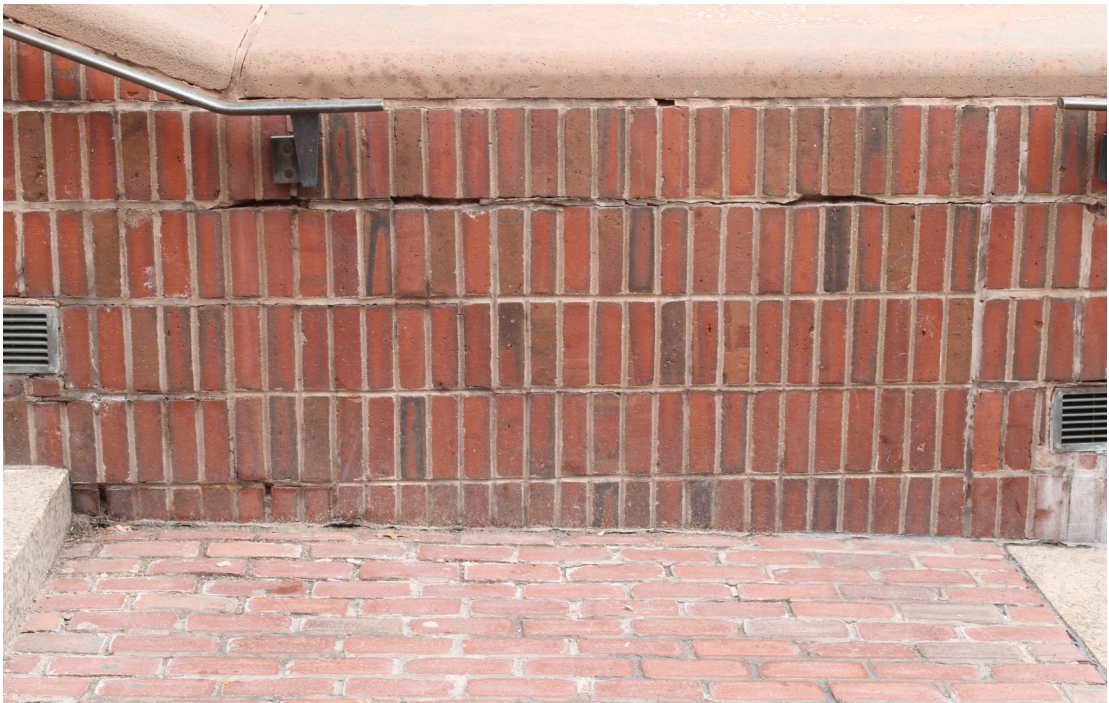
Failed mortar joints (January 11, 2021).
