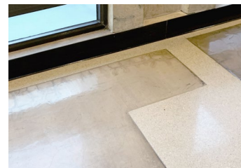
Top: Typical cracking of terrazzo flooring (June 13, 2018).
