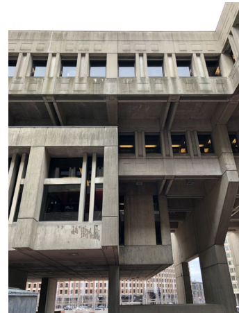
Spalling and organic staining.
