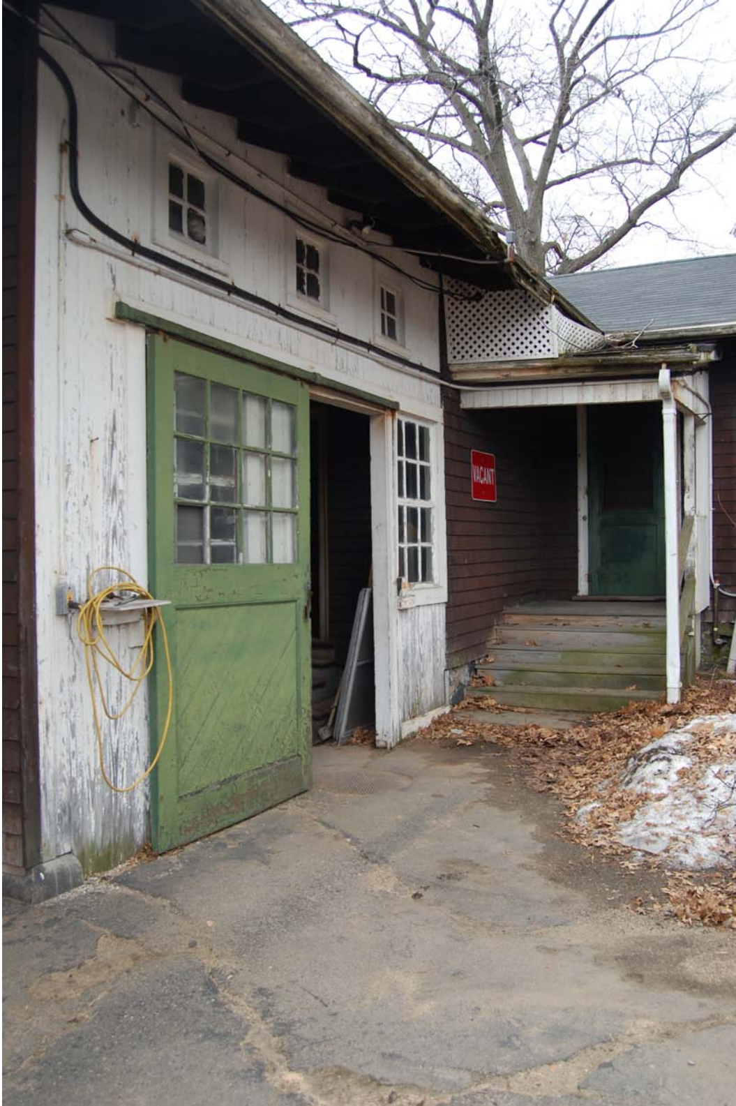
Figure 10. Courtyard-facing elevation of South Shed (C); secondary entrance to Superintendent's Residence (D).
